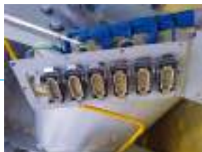
■ High-tension switch cabinet
